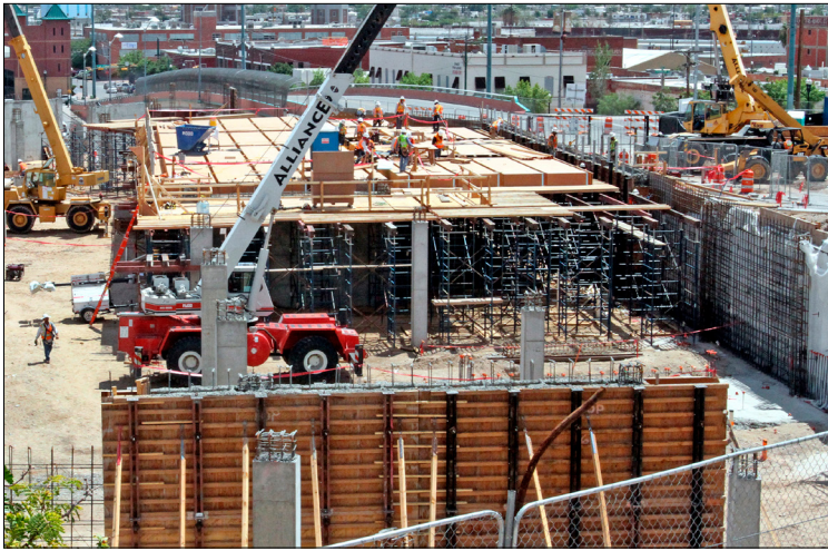
Construction on El Paso's new Triple-A minor league baseball stadium. PHOTO: Courtesy of Rudy Gutierrez and the El Paso Times
