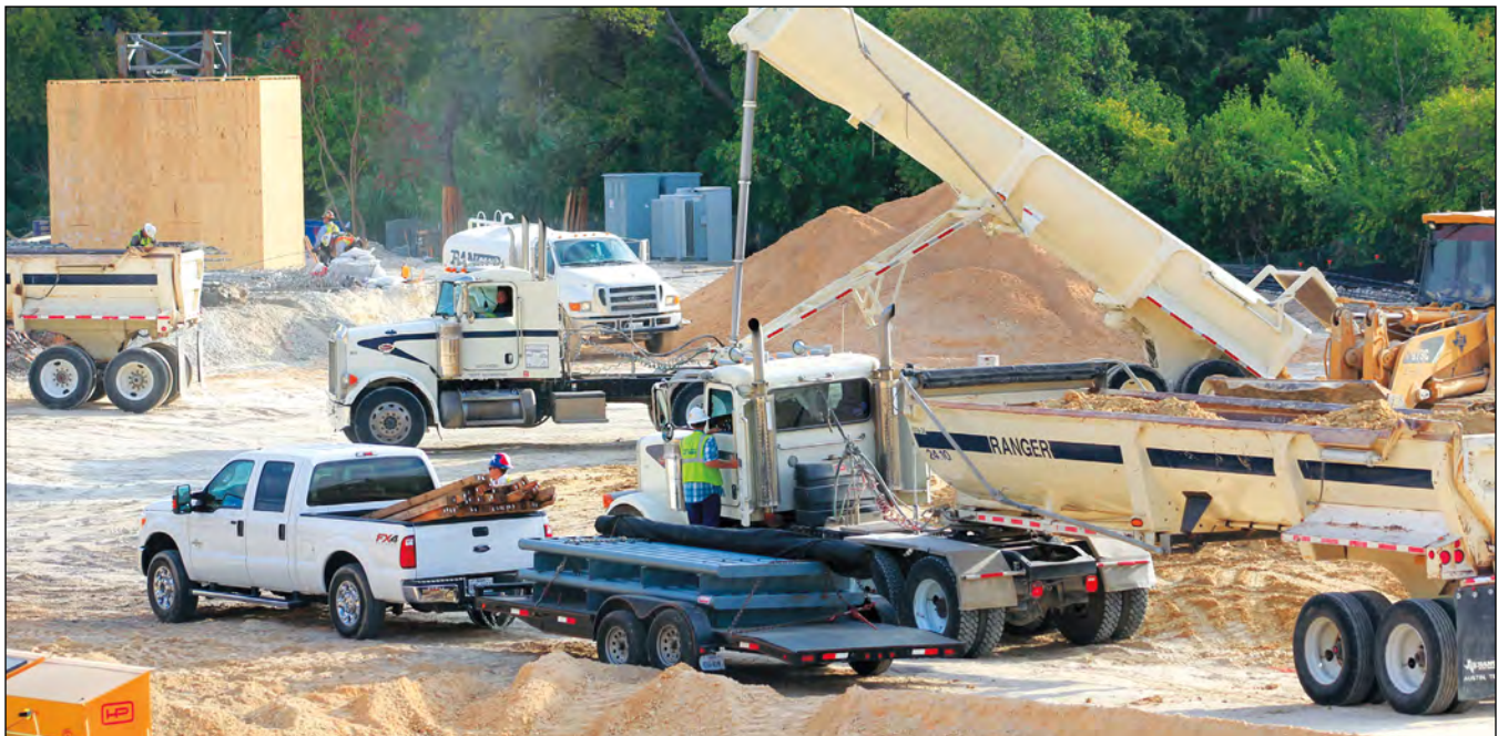
Construction of the Dell Seton Medical Center at The University of Texas. Photo courtesy of Ginger Lowry
